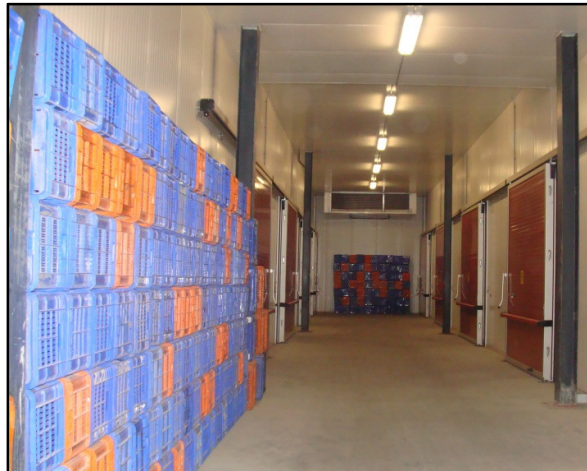
Figure 7: Cold storage corridor at the Long Term Storage Facility in Nagaon Source: OneWorld Foundation India 2013
